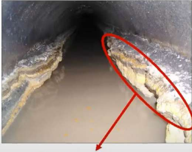
FOG deposits inside of sewer lines
